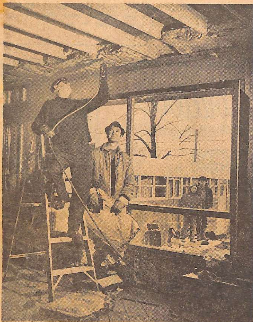
HOME BY CHRISTMAS—The South Windsor Lions Club pitched in during the weekend to help the Robert Bennetts with their new home. Above, Ray Clark, club director, fastens insulation to the ceiling as John Foley of the club's welfare committee prepares to hand him more. In the background in front of the family's bus, which has been home to them since June, are two of the Bennett children, Kenneth, left, and Robert.
