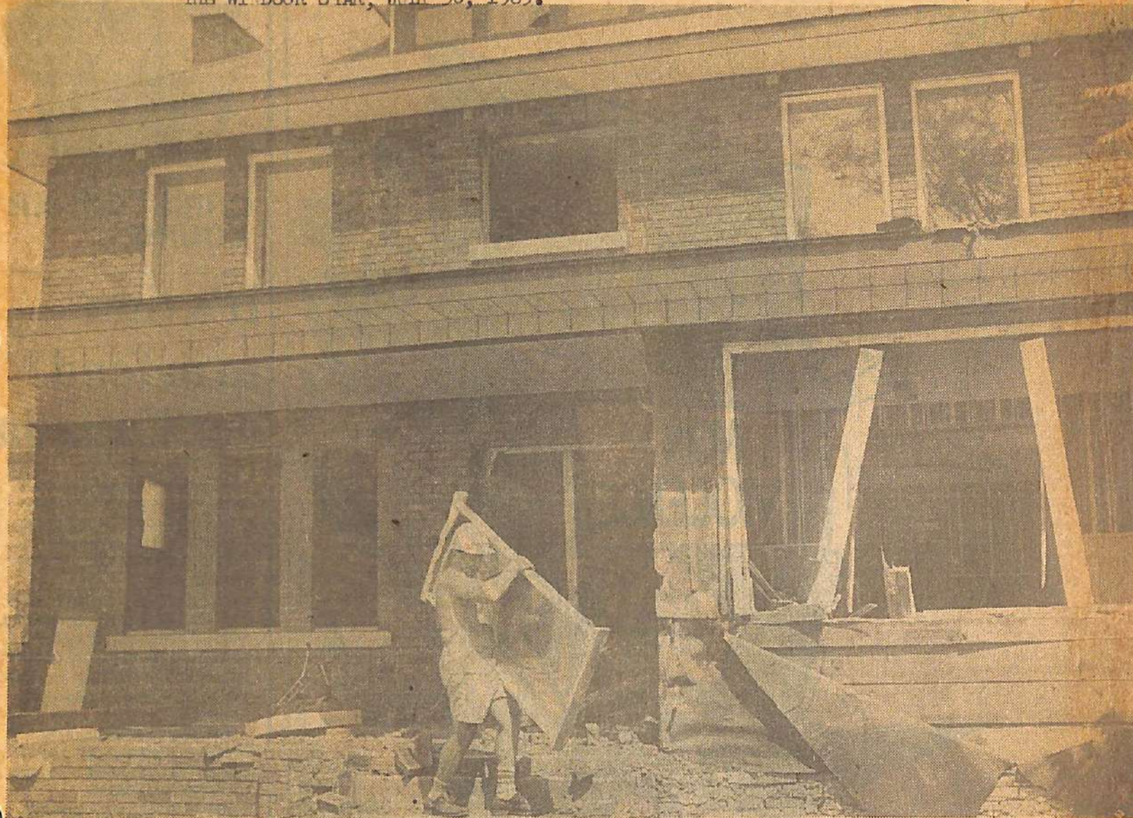
JULIUS VEIGLI of Veigli Construction salvages a window, which would cost $150 if purchased new, from old gambling house
