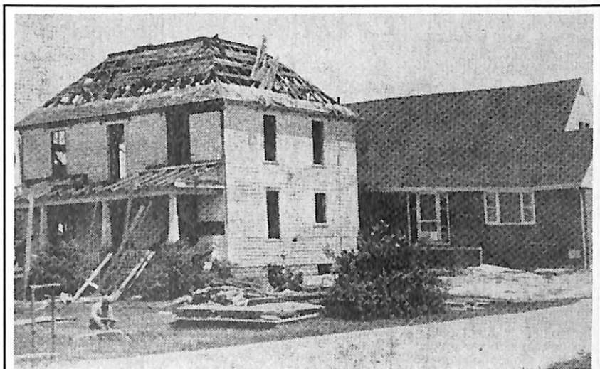
"NEW RECTORY - The old makes room for the new at St. Stephen's Church in Oldcastle where a modern rectory replaces one which has served for "countless" years."
