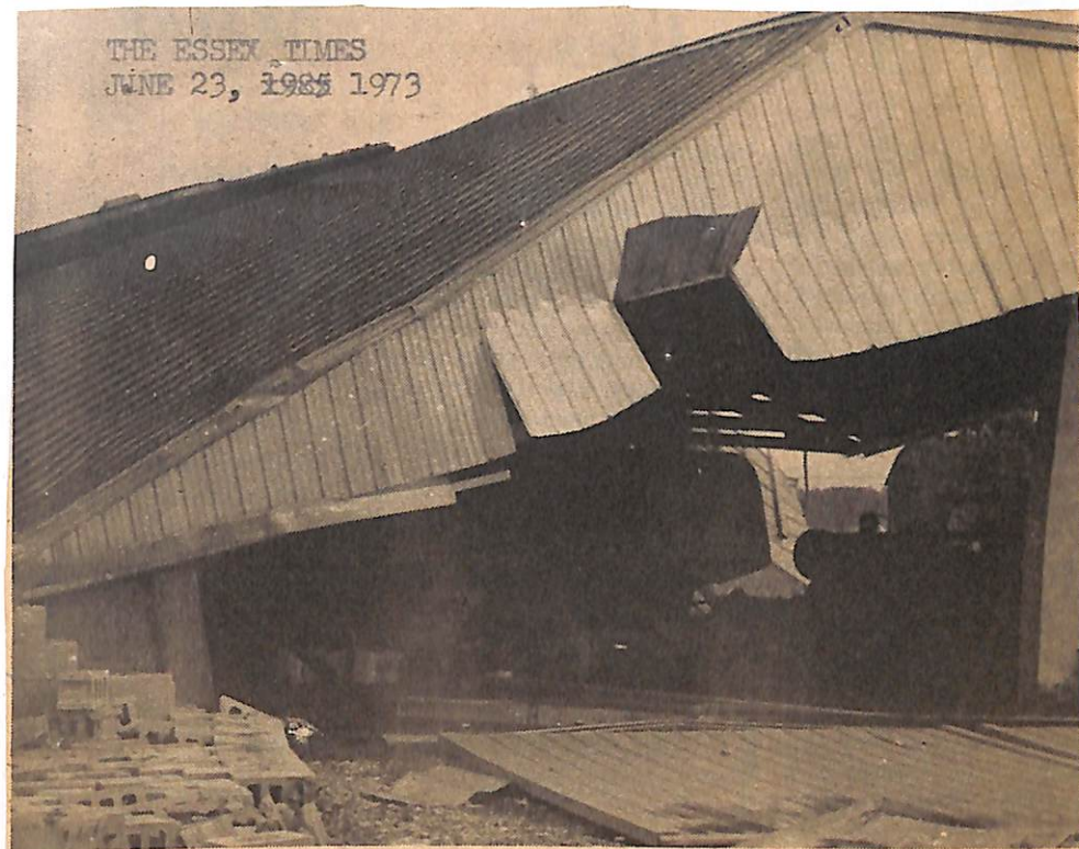
A practically new cement block building was no match for the violent winds on Tuesday night and this building was demolished with farm machinery in it being damaged. This building belongs to Gordon Jobin of the 9th Concession Sandwich South. Also on the Jobin farm another cement block building, a garage and parts of the Jobin home were damaged by the severe winds.
