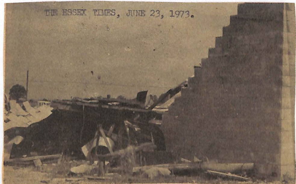
Another view of a cement block building blown down during the Tuesday night wind storm. This building is on the Gord Jobin farm concession 9 Sandwich South. Mr. and Mrs. Jobin were in the house at the time of the storm, but damages to the house were less severe and no injuries were reported.
